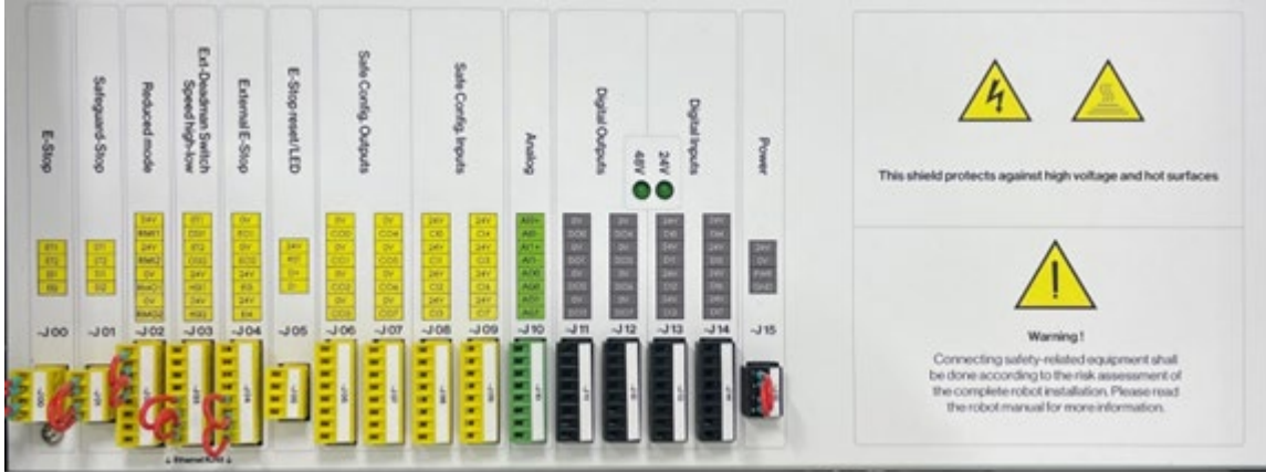
Fig. 26: Default Safety configuration and bridges / jumpers on the Main I/O Board
